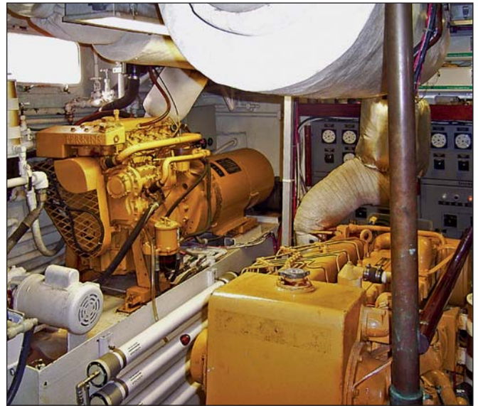
The Oceantide's engine room.
