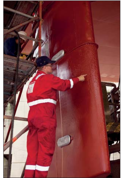
The rudder of M/V Elisabeth Russ in drydock in 2011. No further cavitation damage has occurred in the intervening 7 years.
