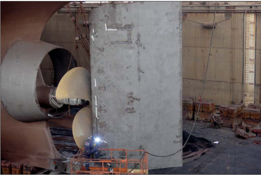
With Ecoshield you will not have to worry about mechanical repairs like this.
