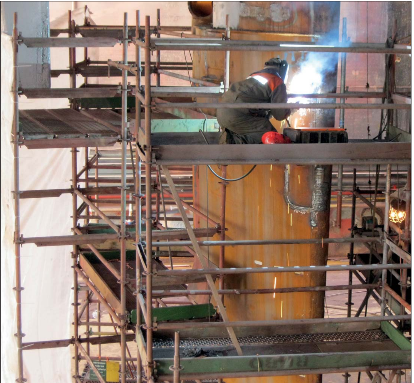
Mechanical repairs like this will no longer be required during future drydockings.
