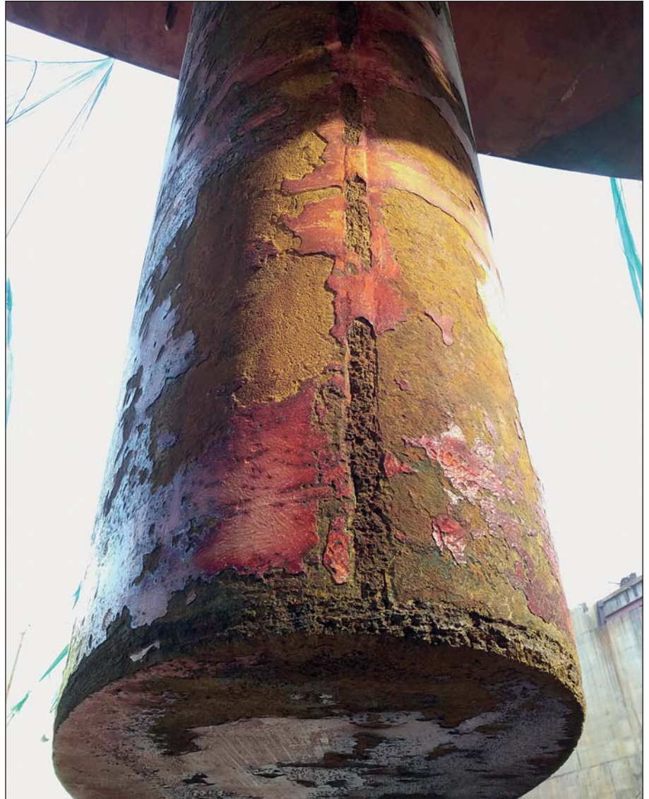
Without proper protection cavitation damage can have a devastating effect on a rudder.
