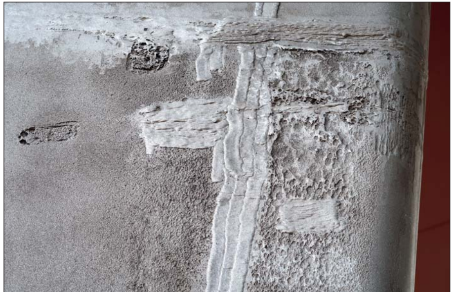
Corroded surface of rudder of ro-ro vessel.
