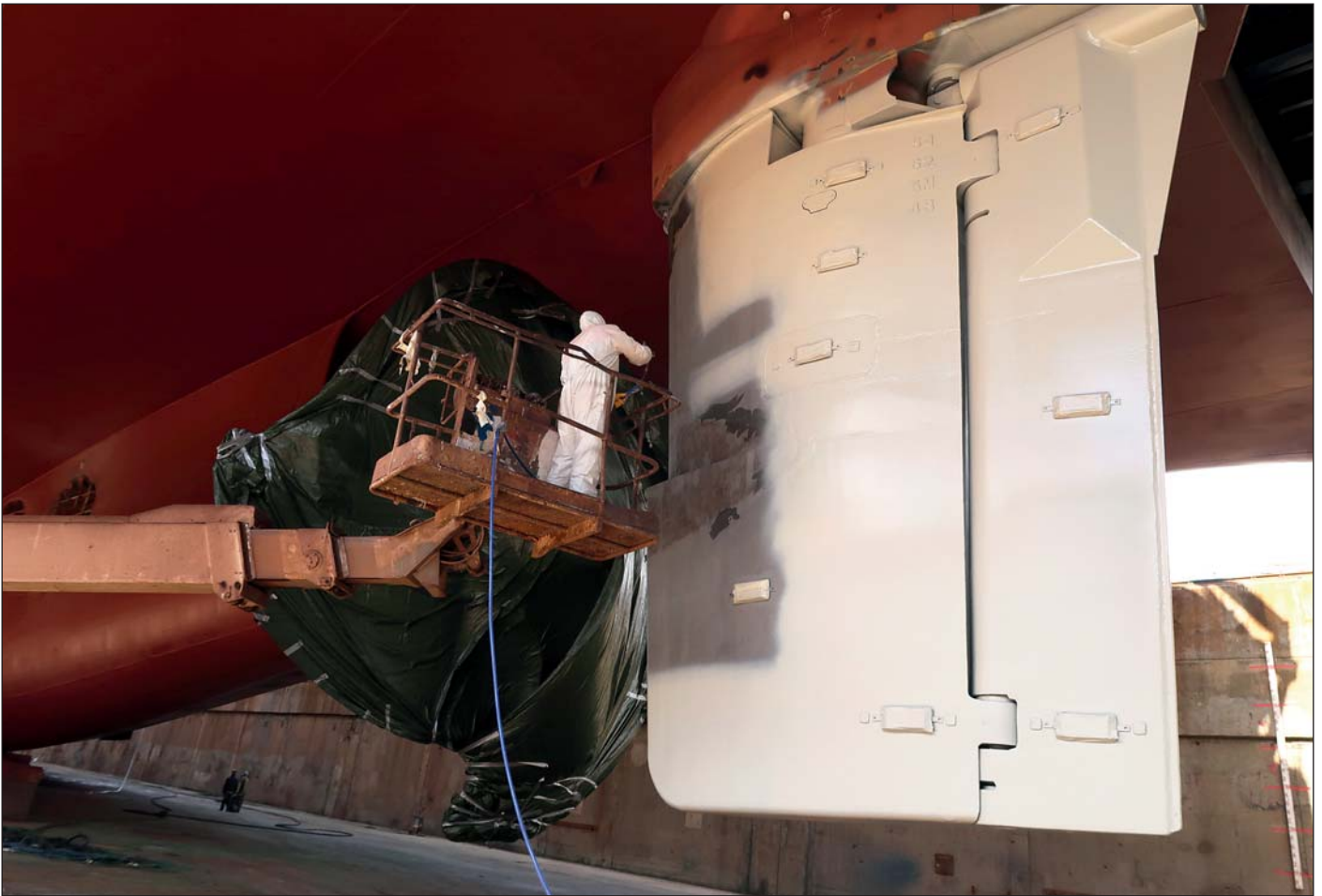
Ecoshield can already be applied one hour after the Ecofix repair was carried out.
