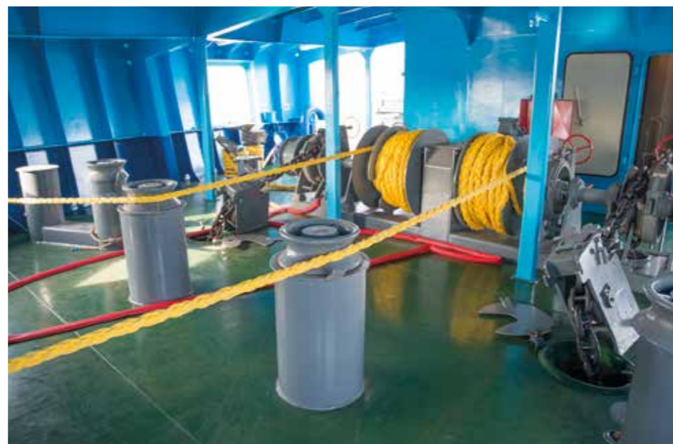
The anchoring and forward mooring equipment is on the enclosed forecastle deck
