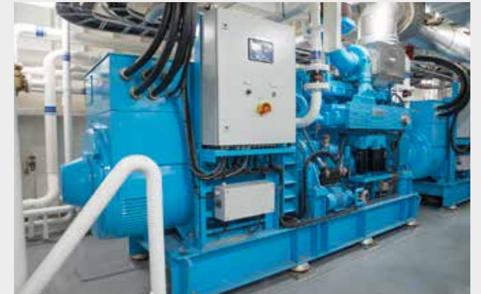
Besides the shaft generator, the auxiliary equipment consists of two main and one emergency generator sets
