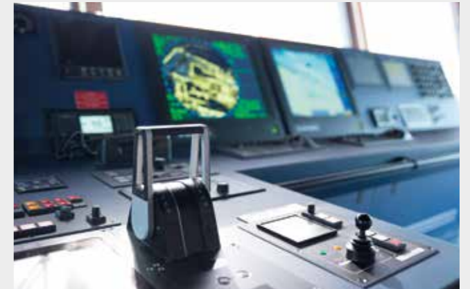
All navigation, communication and ship control facilities are in compliance with Bureau Veritas SYSNEQ-1 notation
