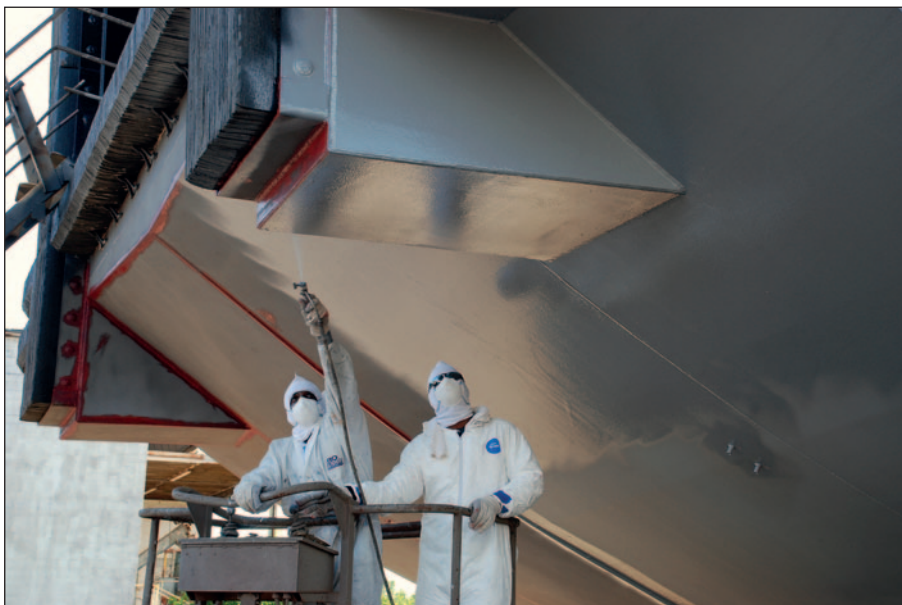
Application of our coatings is very flexible and can be adapted to the yard's schedule.
