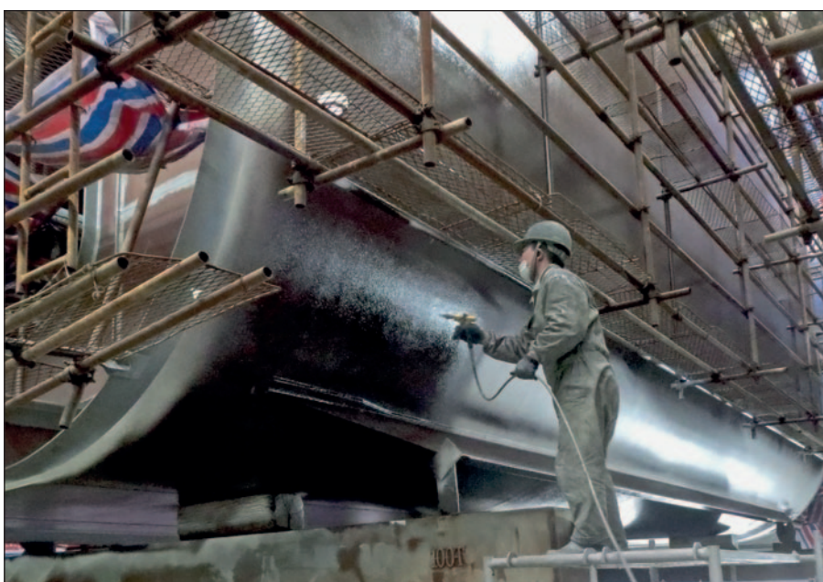
Application of Ecolock on one of the blocks of an EXMAR FSRU.
